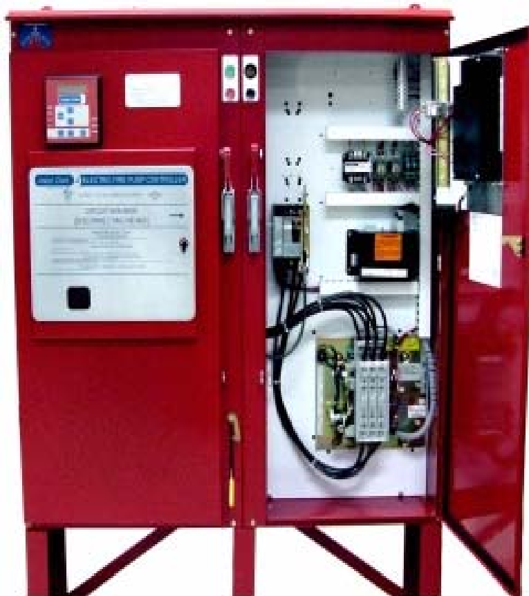
Transfer Switch Controller
